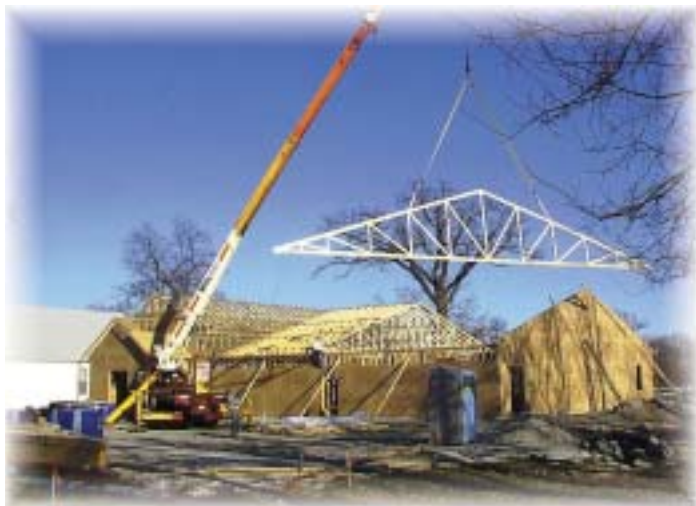
The new space for the Hillsdale (Kan.) Presbyterian Church began to take shape quickly, once the trusses were set.
